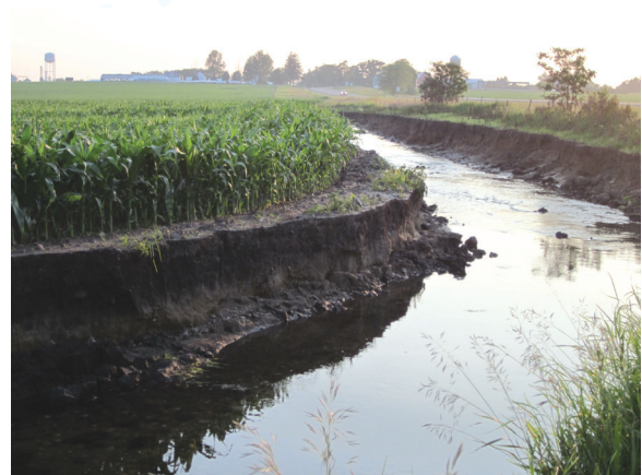
Streambank erosion is a contributing factor to sedimentation in rivers.
